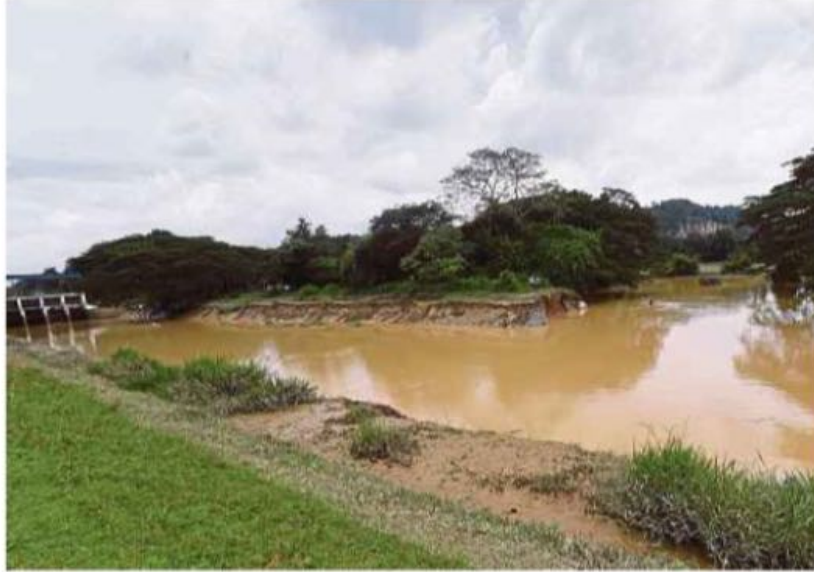
The collapsed bund along the Terusan Tengah irrigation canal near Sungai Bukit Pinang in Pokok Sena, Kedah, yesterday. BERNAMA PIC
